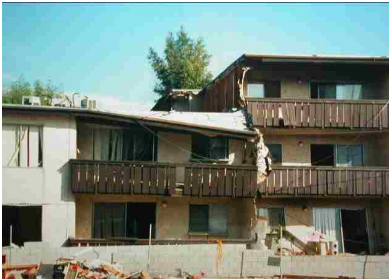
Figure 4-3: Differential settlement splitting an apartment building (after Friedman, 2007).
